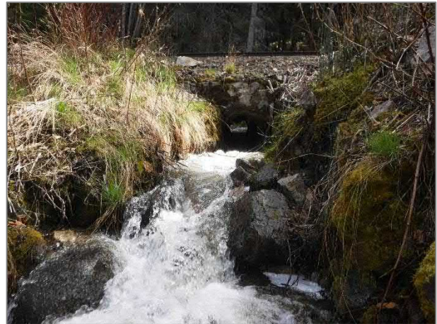
Photo 4. Bose Creek culvert under railway.
